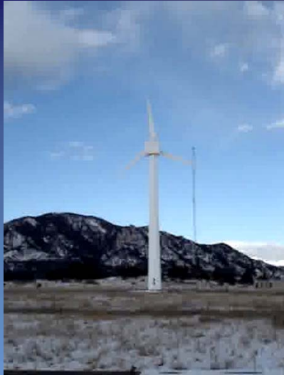
15 Meter Diameter and 100 kW
